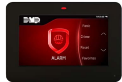
Screen Turns Red in Alarm
